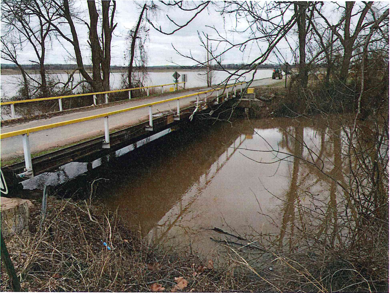
Figure 6 Flooding in the Lollie Road area
