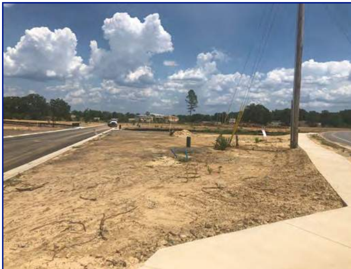
View of subject property from Tsar Rd @ Bill Bell Ln looking E
