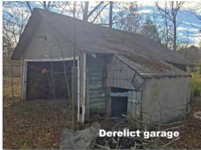
Accessory structure to be removed
