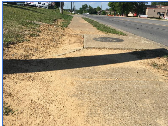
Example of a sidewalk that is uneven and not fully accessible
